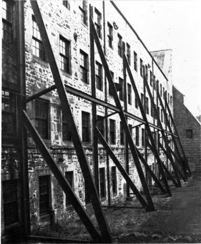
Page 108 (left) Rear of No 1 mill. The steel reinforcing was added when the mill was cut down to stop it falling into the river Clyde; (below) rear of mills 2 and 3 with the School in the background and preparation rooms on the right
